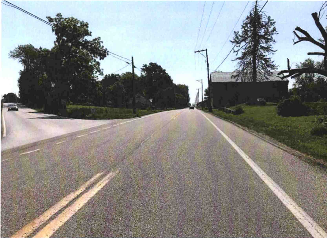
Direction / Road: EB York Road (SR 0074) Approach / Departure: Approaching Shughart Road Distance: 50 feet
